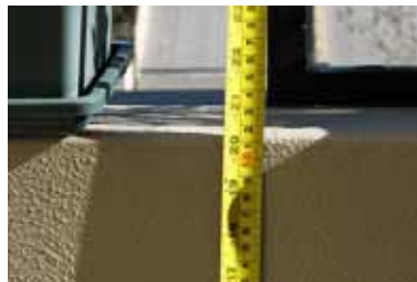
Photo No 81 (Unit 301 SW balcony balustrade)
