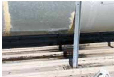
Photo No 107 (exhaust duct leak)
