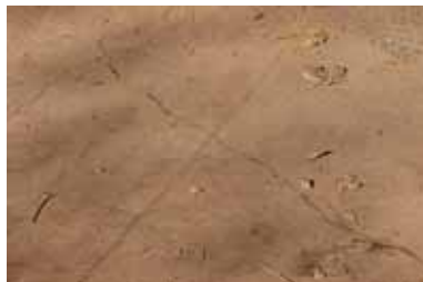
Photo No 91 (driveway hairline cracking)
