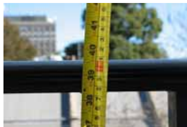
Photo No 81A (Unit 301 SW balcony balustrade)
