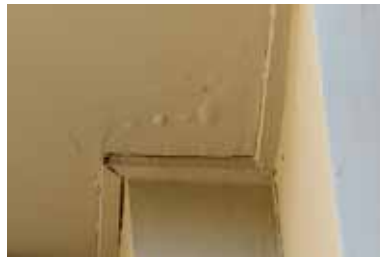
Photo No 88A (sample balcony soffit leak damage)
