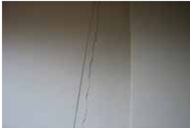
Photo No 76 (unit 107 drummy balcony render)
