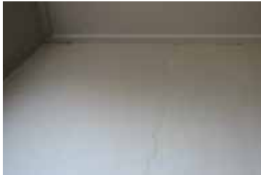
Photo No 75 (unit 107 balcony falling damp)
