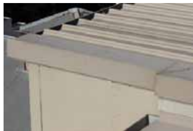
Photo No 108 (SE corner parapet leak)
