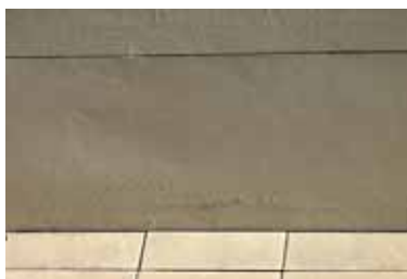
Photo No 84 (Penthouse western balcony damp)
