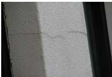
Photo No 77 (cracked external render/paint)
