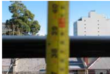
Photo No 80B (Unit 301 NW balcony balustrade)
