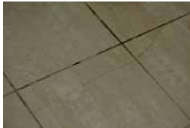
Photo No 74 (unit 302 cracked bathroom tiles)
